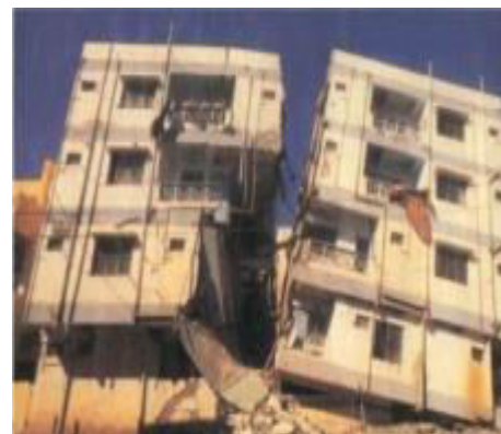
Figure 1: Damage of MI RC building amid 2001 Bhuj Earthquake
